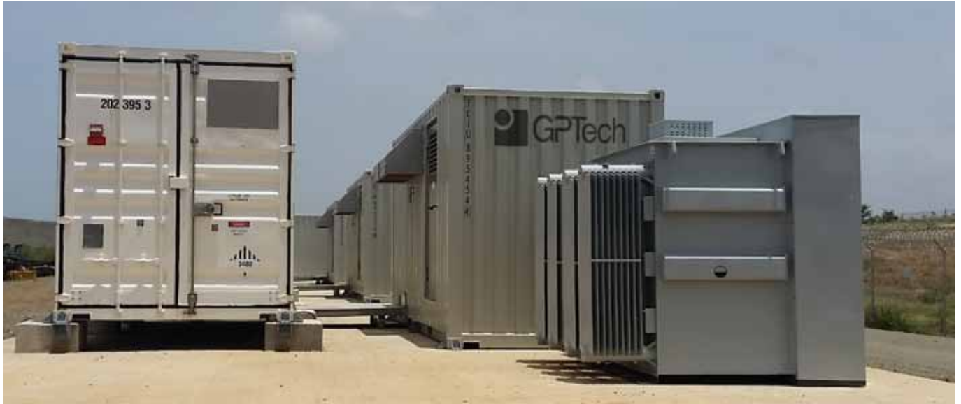
Complete Storage Systems , the two main elements (BESS and APCS) and the MV transformer
