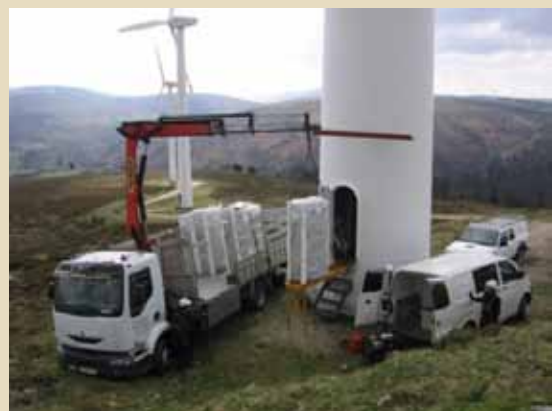
2008: GP Tech STATCOMs installation for a 50 MW Wind Facility in Spain
