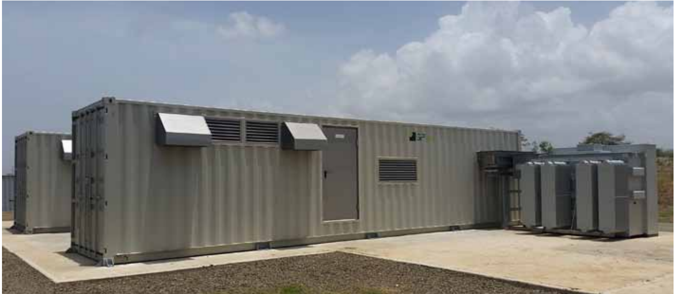
STATCOM systems installed in the facility , integrated in two fully-aconditioned 40ft maritime containers
