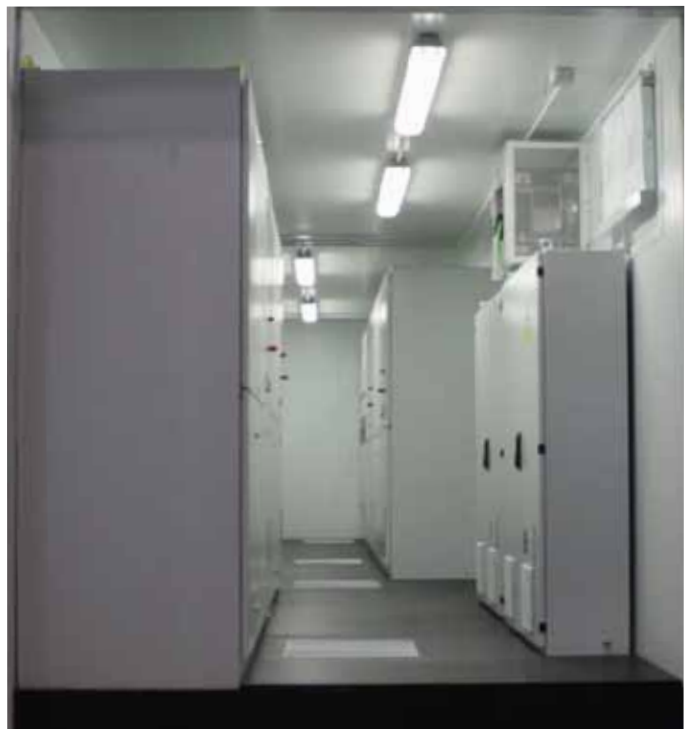
Inside the AVCS , 4 SVC1000 are installed with customised aconditioning systems and all the protection and auxiliary components
